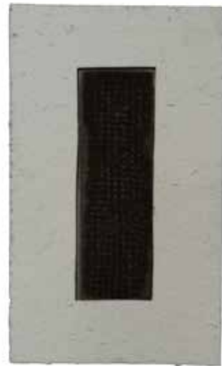
Burner with face insulation in place
