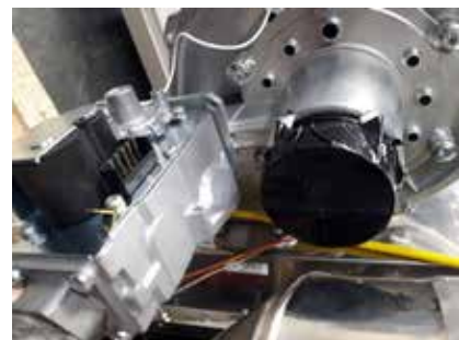
Large venturi covered with tape
