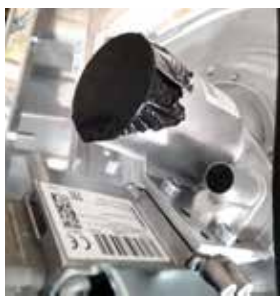
Small venturi covered with tape
